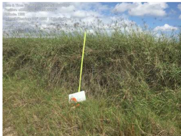
7532 - Bank Erosion, Interior
