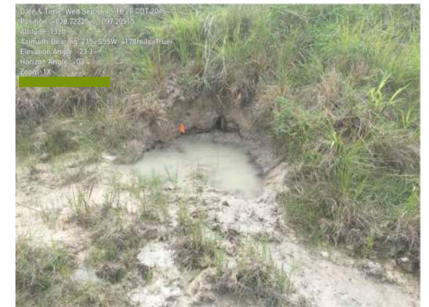
7470 - Exterior Toe (Wet/Erosion Area)
